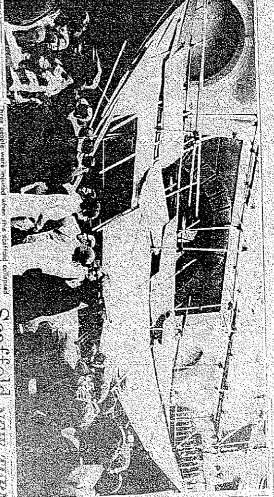
Three people were injured when this scaffold collapsed in Kingsley Street Johannesburg yesterday. A crowd of onlookers gathered to see the wreckage.
